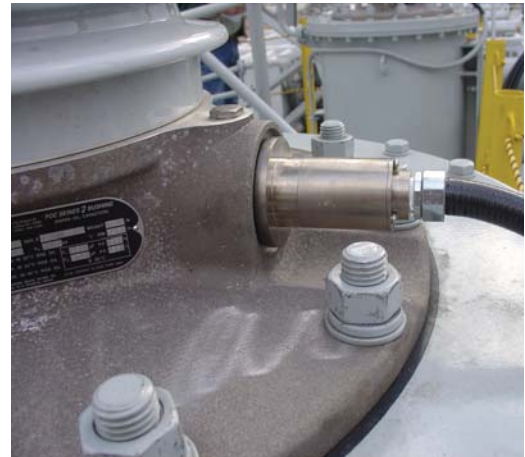
(b) Sensor installed in bushing test tap
