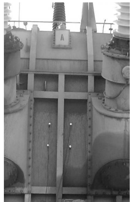
Figure 10 – Acoustical sensors installed on transformer tank
